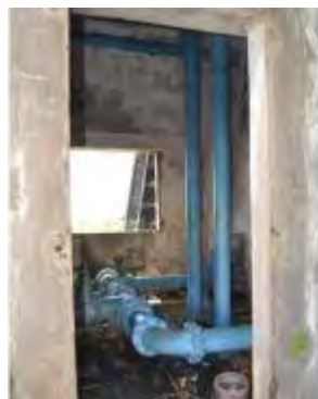
Figure 13-20: SEG Water Pumping Station and Water Tank (view from inside) adjacent to the Project site
